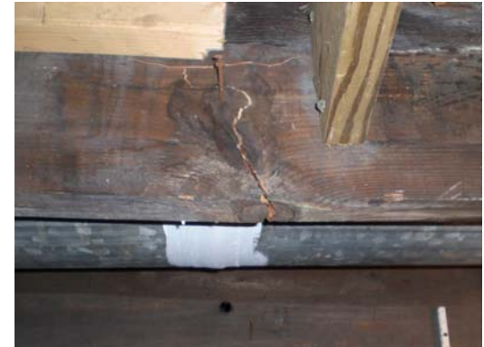
Cracked floor Joist from age and excessive settlement
