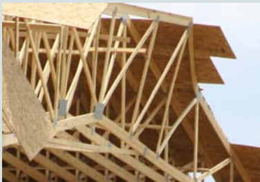
Failed roof members
